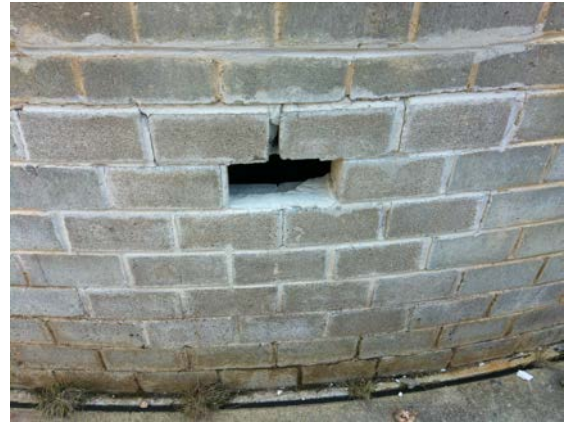
Image 11 Another missing brick at observatory (ACT Heritage 2015)
