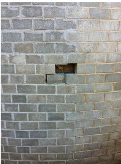
Image 10 Missing brick at observatory (ACT Heritage 2015)
